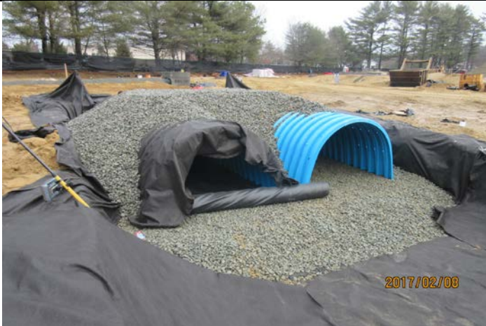
Infiltration System at Play Area
