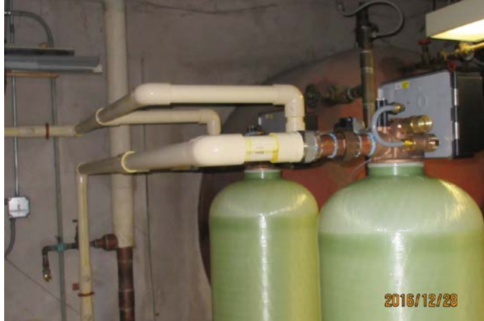
Temporary Water Treatment System
